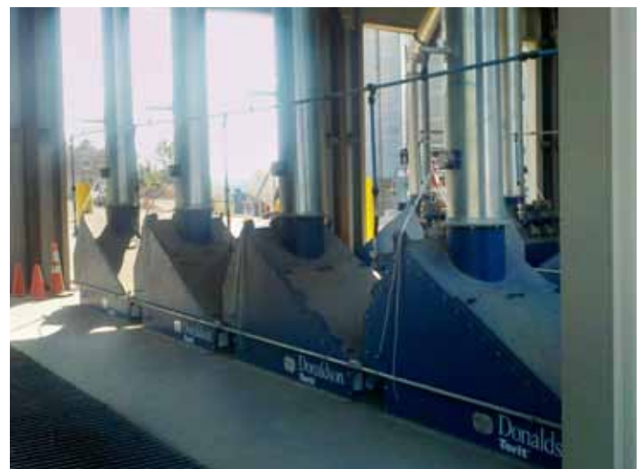
Four Donaldson Torit CPV-6 collectors at grain truck dump pit.
